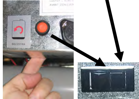
Location of switch on an electric fryer is behind the far right control box.
